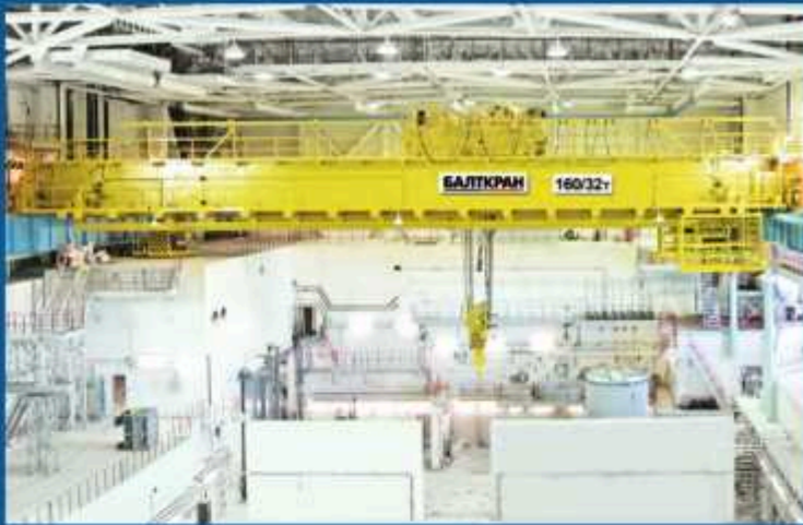
LENINGRAD NUCLEAR POWER PLANT-2, SWL 160 T, SNF WORKSHOP
